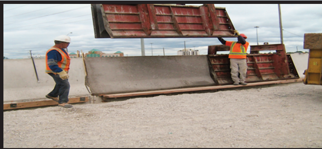
Figure 4. Bridge walls cured in less than two hours in subzero temperatures in Ontario, Canada. Credit: NanoArchitech.
